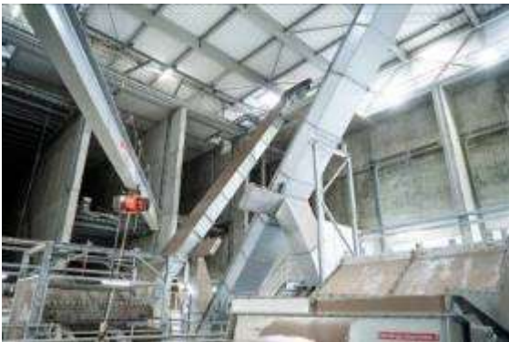
Image 2: The conveyor system then transports the material into storage boxes, en route to which an over-the-belt magnet frees the fuel from metal objects like screws and nails.
