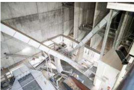
Image 3: Vecoplan supplied all the machinery for the plant and took responsibility for its assembly and commissioning.
