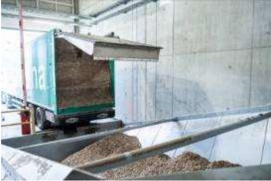
Image 1: The truck unloads wood chips, fresh from the forest, onto a drag chain discharger. The unloading process takes about 15 minutes.
