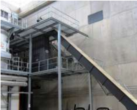
Image 7: A drag chain conveyor transports the biomass to the boiler.
