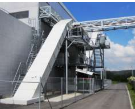
Image 3: Vecoplan supplied a tailor-made storage, dosing and transport solution. Scraper chain conveyors are an important element of the solution.
